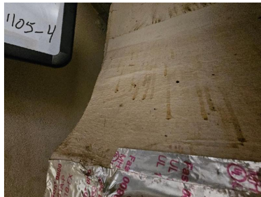
1105-4 Duct Mastic Typical Interior HVAC
